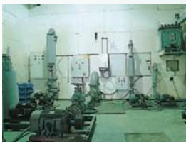
Testing area for Roots Blower
